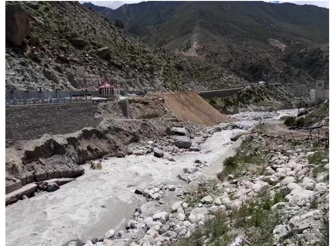
Partial river Embankments were washed away
